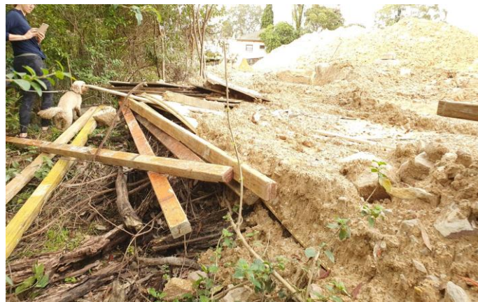
Next to the Angophora is this pile of building materials which has been washed downslope and will now be trashed by builders – they are obviously not even adequately containing their own materials.
